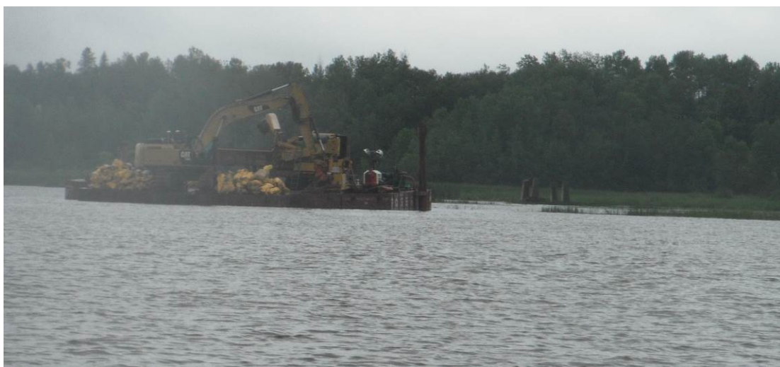
Figure 20. Active restoration to remove bottom sediments at Radio Tower Bay in St. Louis River Estuary. NRRI sampled this site in 2011, but could not resample in 2015 due to continued restoration activity. It will be important to re-visit and collect more data within the next round of CWM sampling.
